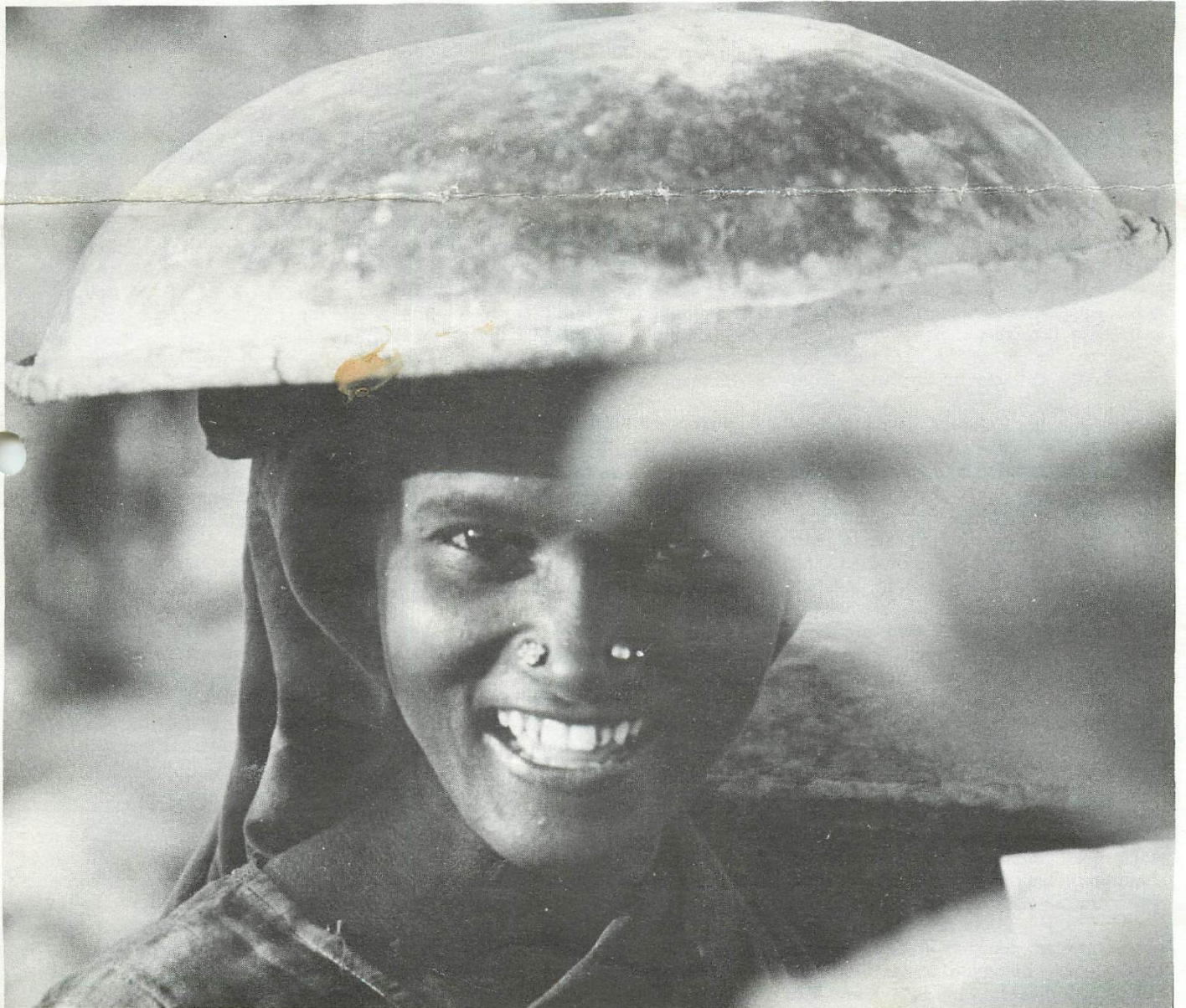
A young Indian girl, working on the construction of a dam, returns for more concrete with her pannier upside down on her head.
