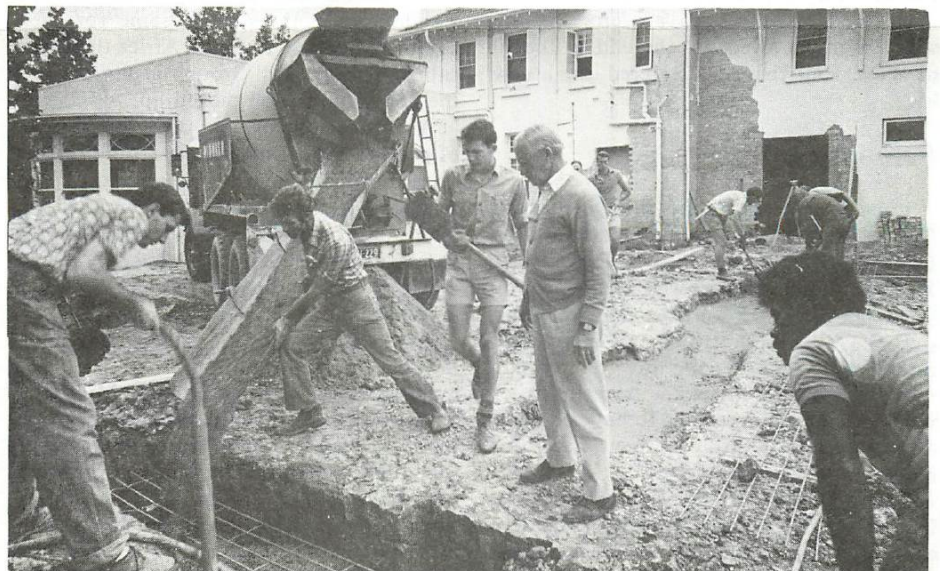
Foreman Vin Russell pours foundations watched by Gordon Brown, architect, and assisted by other voluntary workers. Mr Brown donated his architectural services. Photo: Mayor
